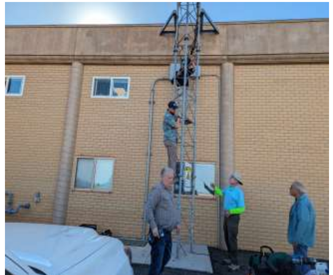
Austin (W1EPR) and Mike (KI7ZXC) on tower pulling coax through the wall to connect to the antenna.
