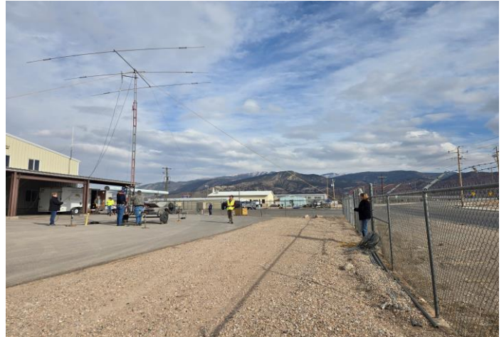
Antenna Tower is coming down. Ann (KJ7OGZ) on right against fence holding guy rope.
