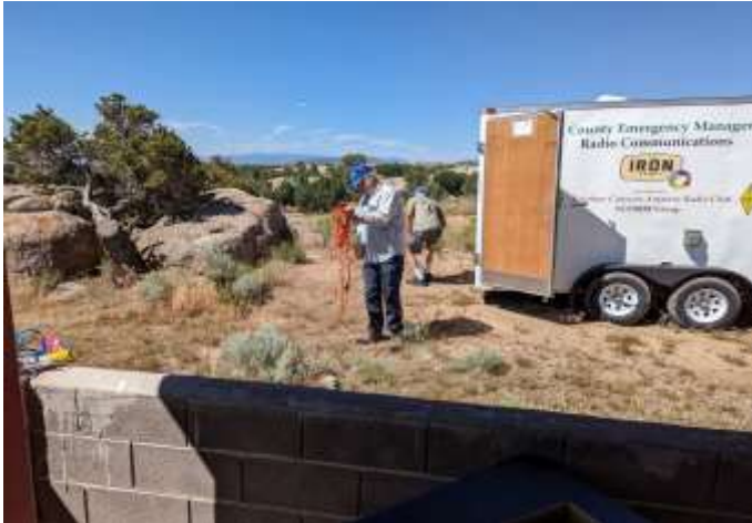
Fred (K17TPD) bring power in from the generator left of the trailer down in the valley.
