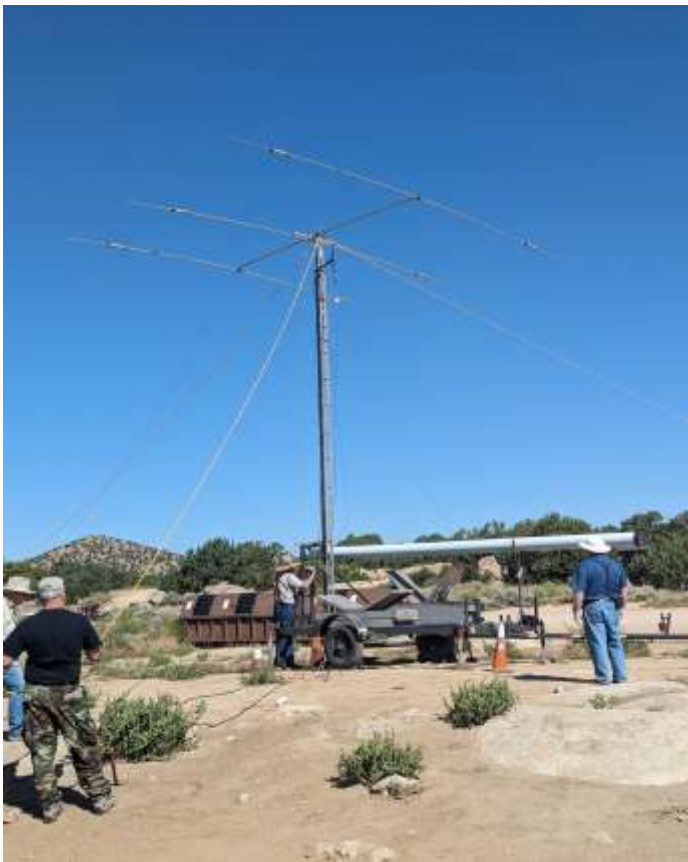
First section of the mast is up. Volunteers checking everything before mast is raised further in the air.
