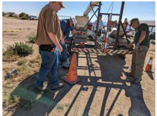
Brody (K7VXV), Dick (K7ZI) and Bruno (KG7VVN) checking the trailer level prior to antenna install.
