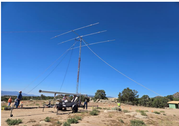
The tower is up and the 2 nd session is being raised. The trailer will then be secured with the guy ropes etc. for use.
