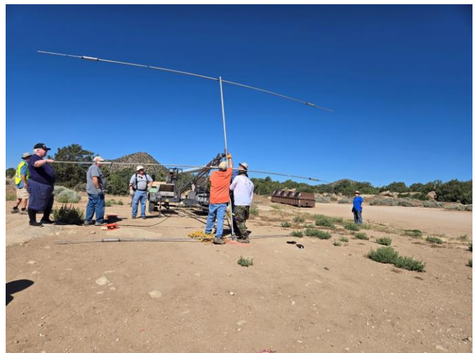
Brody (K7VXV), Kevin (K2MFK) and Fred (KI7TPD) attaching antenna to the tower before tilting the tower upright.
