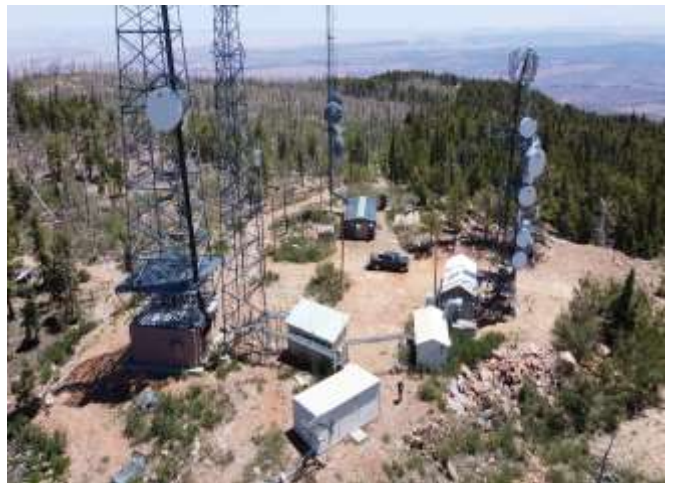
Aerial view of the Navajo Repeater Mountain Site. Intertie building bottom (Center) of picture
