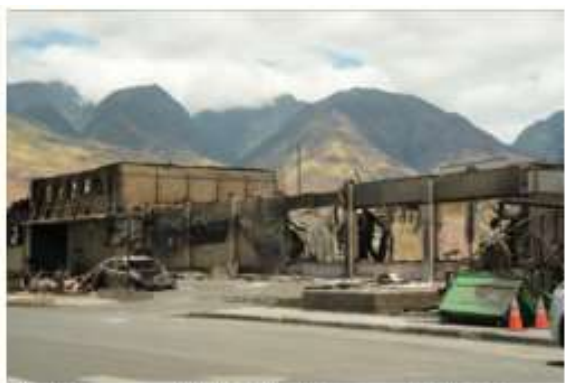
Fire Damage at Wailuku, HI (Dominick Del Vecchio/FEMA, photo)
