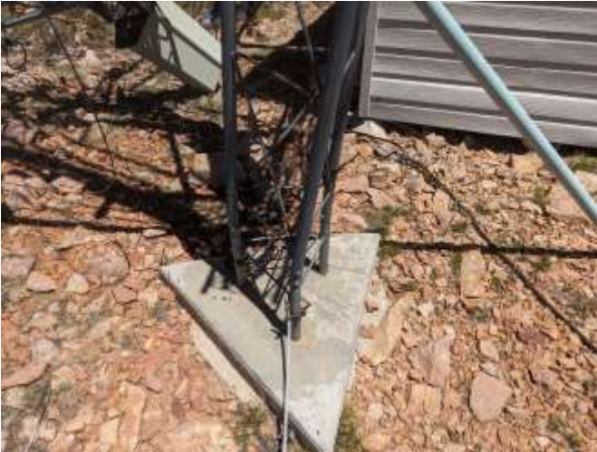
Tower legs are bent by cement platform.
